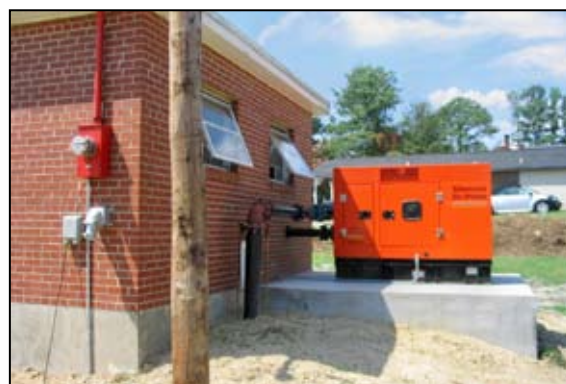
Permanently installed Dri-Prime pump at Edenton, NC.
