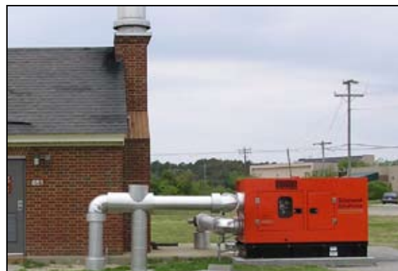
Permanently installed Dri-Prime pump in Fort Story, VA.
