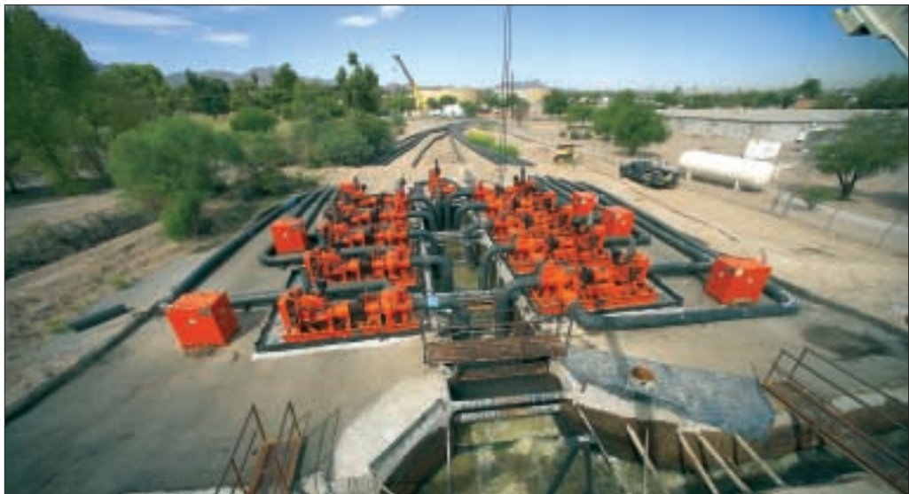
Godwin is known for complex bypass projects such as this 105-mgd bypass using 16-in. Dri-Prime pumps in Tucson, Ariz.
