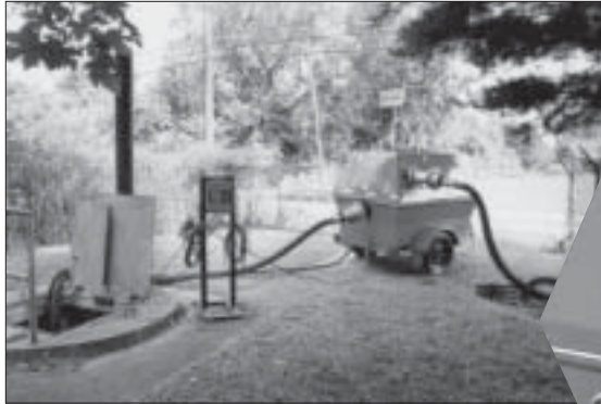
Municipal Pump Station Bypass
