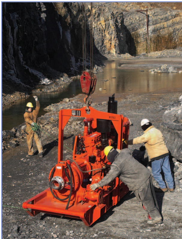
In preparation for dewatering, installers set in place a 6" x 4" Godwin high head Dri-Prime® pump which will move up to 295 cubic metres per hour or 1,300 US gallons of water per minute.
